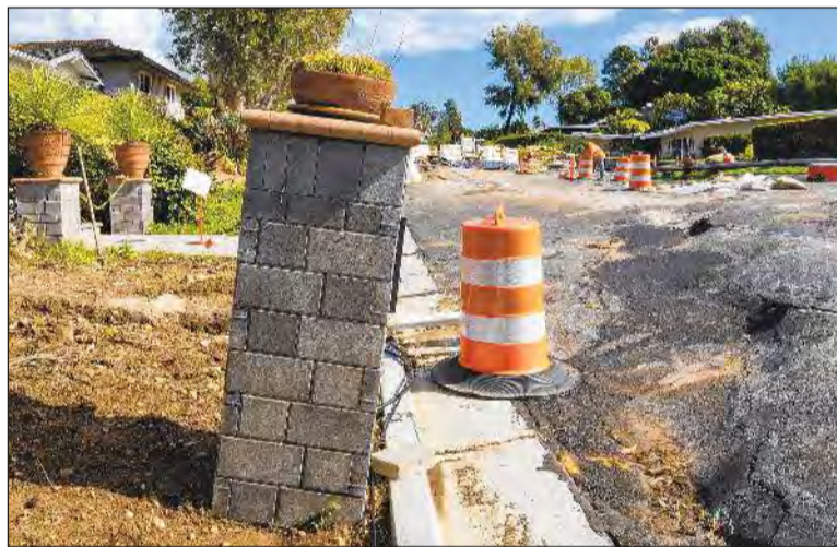
A MAILBOX in the Seaview neighborhood is askew after land movement exacerbated by recent storms damaged homes.
